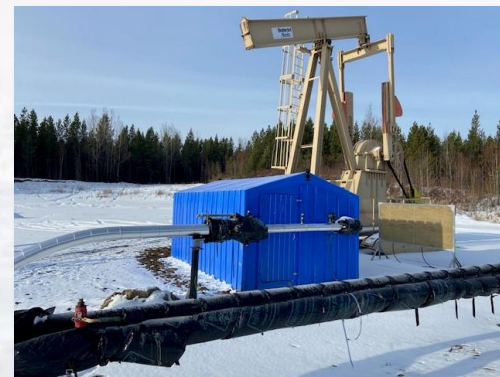
1-4 old pump jack and new well shack
